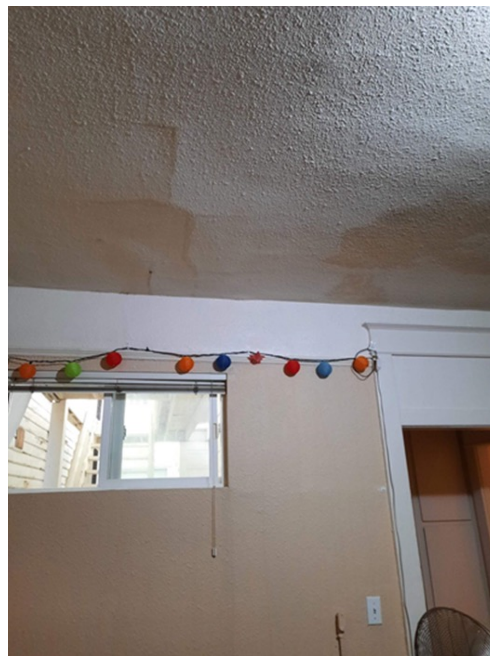
Above: Photo Credit - Ogden, Ruth. (2021). Water damage in my apartment ceiling. Personal Collection.
